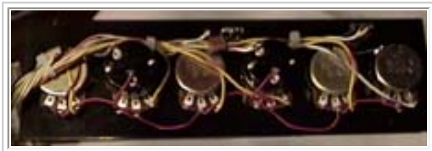
Rear view of the front panel showing the wiring of the potentiometers.
